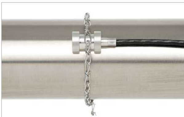
PT100 transducer fixed to pipe
